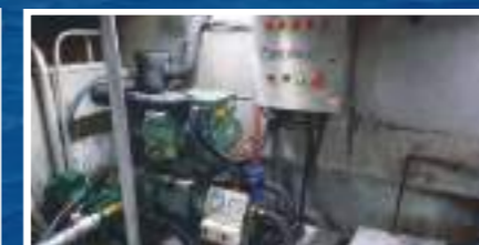
Compressor unit installed inside engine room
